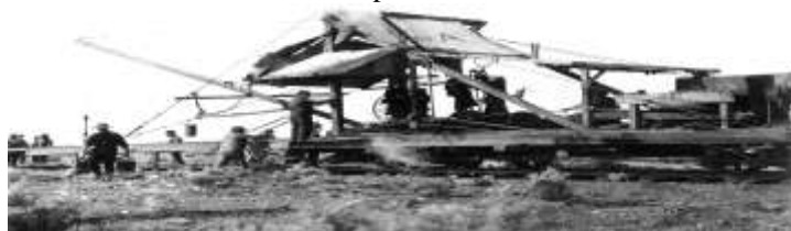
Tracklayer used during the construction of the railway line across the Nullarbor Plain
